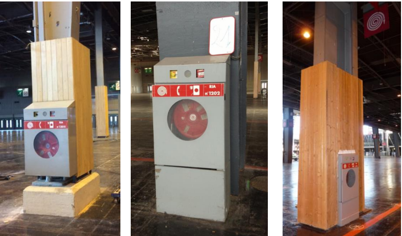
FIRE HOSE REEL
