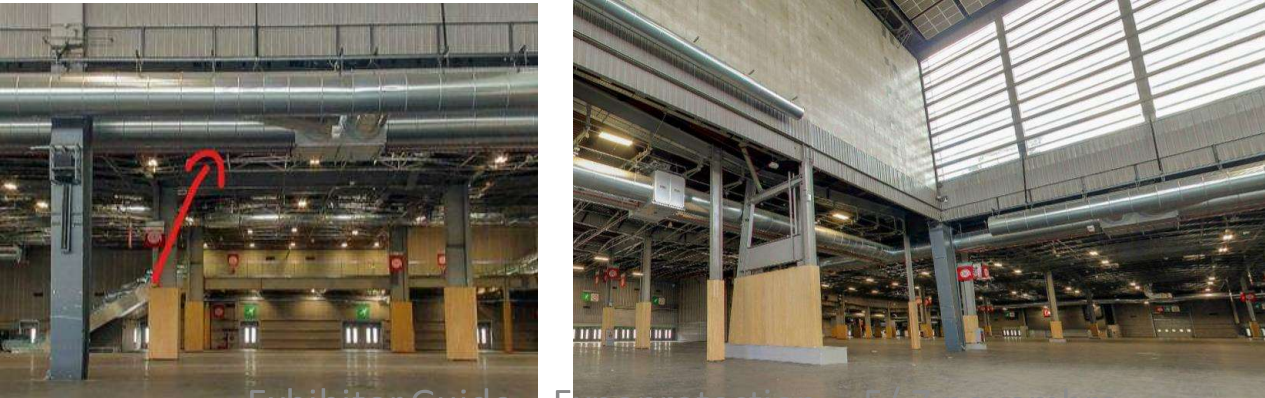
CEILING AIR CONDITIONING DUCT (requiring a feasibility study from Viparis if you wish to sling a structure)
