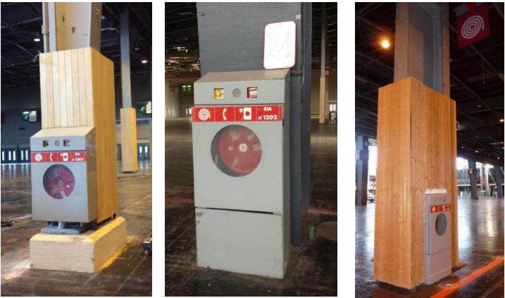
FIRE HOSE REEL
