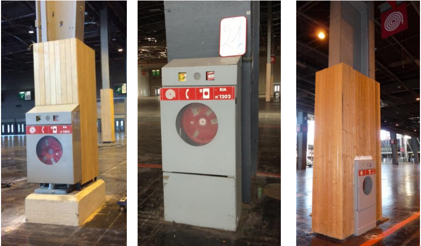
FIRE HOSE REEL
